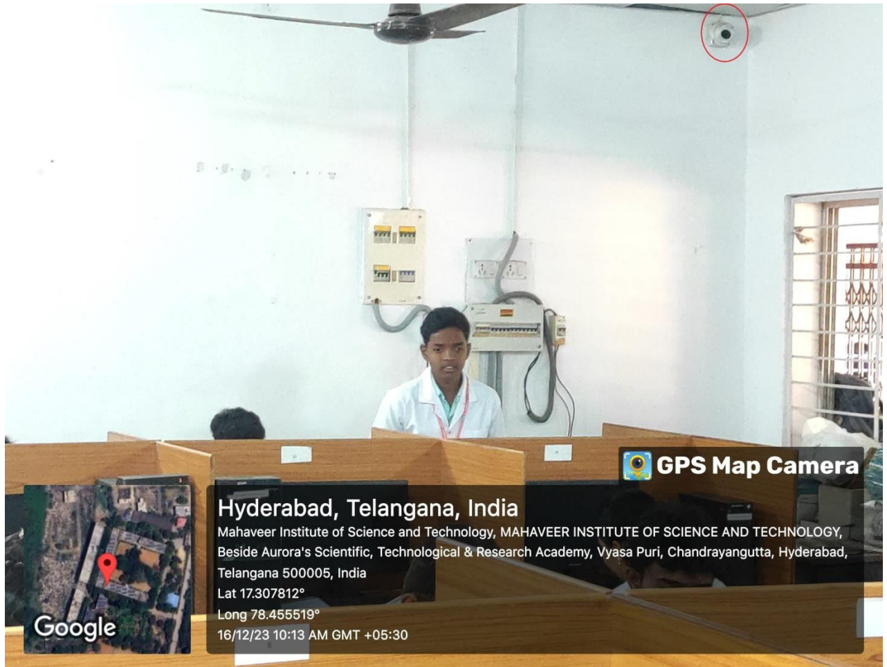
ii. Camera Installed in Every Lab
